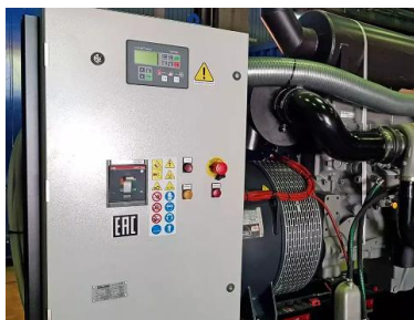
Figure 2. External view of the automatic transfer switch (ATS) for a diesel generator set
