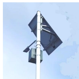
Figure 6. Lighting pole with a complete set of equipment for autonomous lighting
