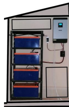
Figure 8. Battery bank configuration for the electrical installation
