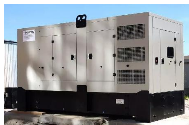
Figure 3. External view of the DGS-200 diesel generator set in an enclosure configuration
